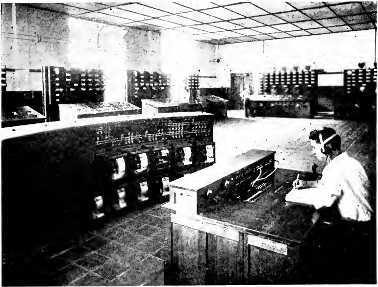
FIG. 376.—Mississippi River Power Company. Chief Operator's Room Showing Control Boards and Switchboards.
